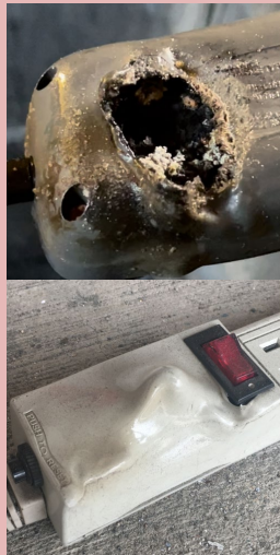
Melted power strips: Top: sum of devices > capacity Bottom: single device > capacity
